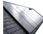
Solar PV panels
