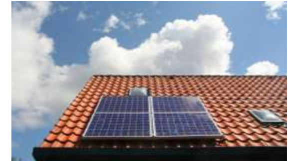
EXAMPLE OF DOMESTIC SOLAR PANELS ON ROOF
