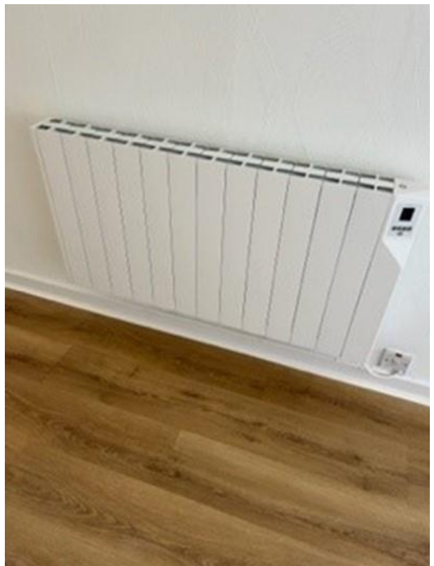
New Electric Heaters
